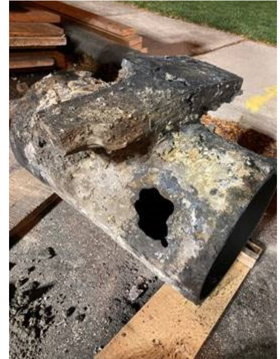
Part of an old leaking main
